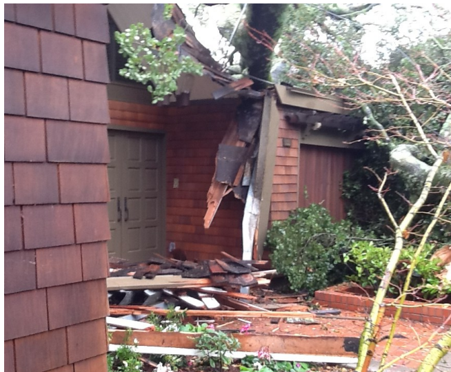
December 11—Storm damages & flooding, San Mateo
